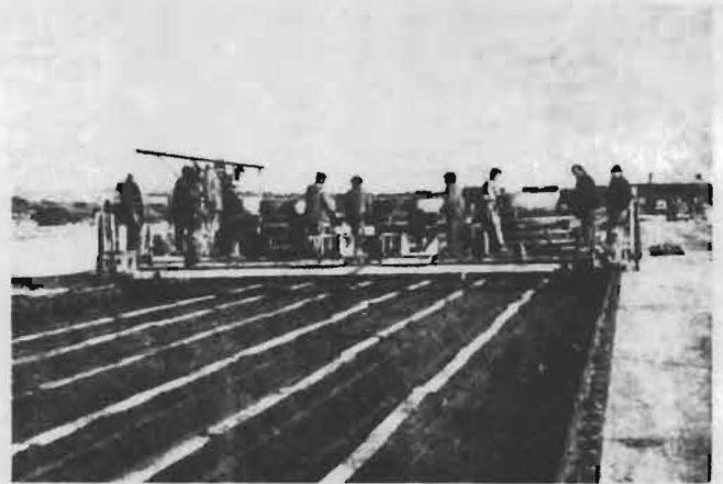
Fig. 5—Installation of prestressing steel; the wire-laying machine places about 20 tons (22 U.S. tons) of prestressing steel in the longitudinal direction when running between two abutments of a prestressing strip
