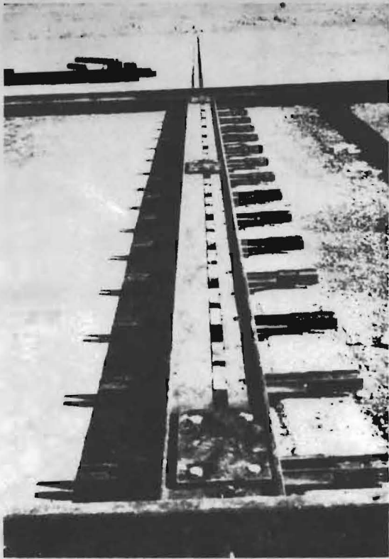
Fig. 7—Built-in tensioning joint; this type of joint is placed between two prestressing fields; it is installed on the abutment; the steel plates situated vertically between the angles transmit the anchorage force of the tensioned wires in the prestressing field (not yet installed in the photograph) from the joints to the abutment
