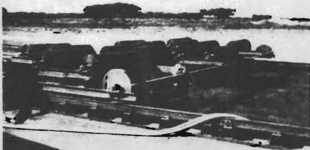
Fig. 2—Paper-laying machine; running once over the prestressing strip 5000 sq m, this machine places the total quantity of paper for separating the slab and sub-base; there are two layers of paper of 180 g per sq m (5.4 oz per sq yd)
