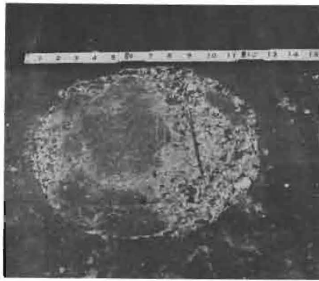
Figure 6. Failure in top surface of slab 2.
