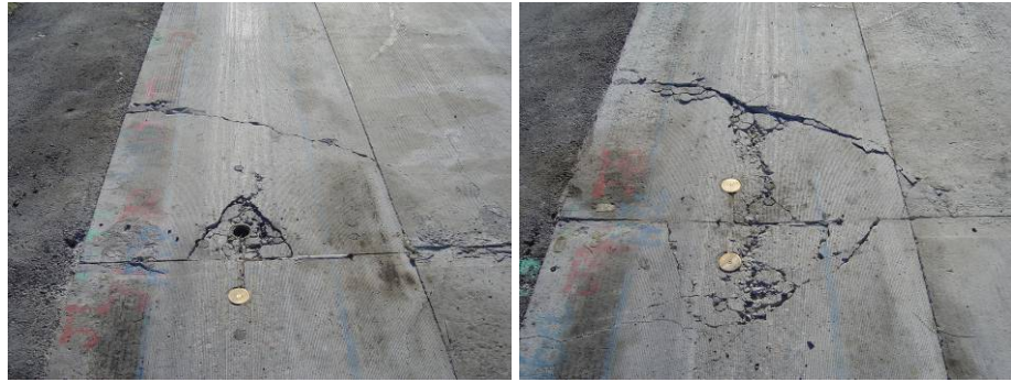
Figure 16. End of life at the two joints of section 1, loaded to failure.
