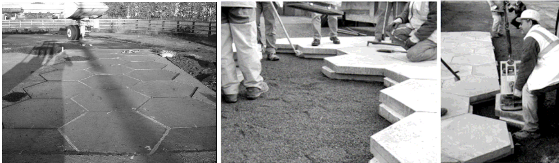
Figure 4. Accelerated pavement testing of hexagonal slabs and installation of keyed slabs in France (13).
