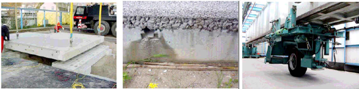
Figure 2. Construction of the ModieSlab test section for accelerated pavement testing and the LinTrack facility (9).
