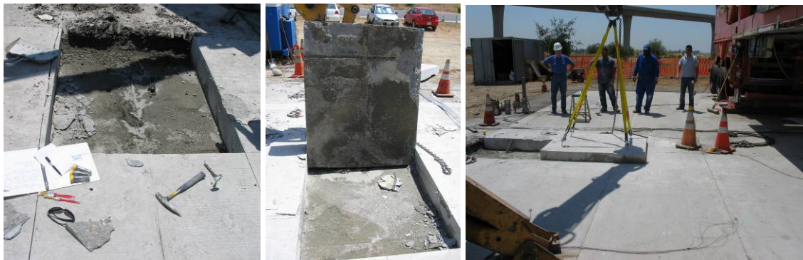
Figure 14. Investigation of void under the slab in section 2.
