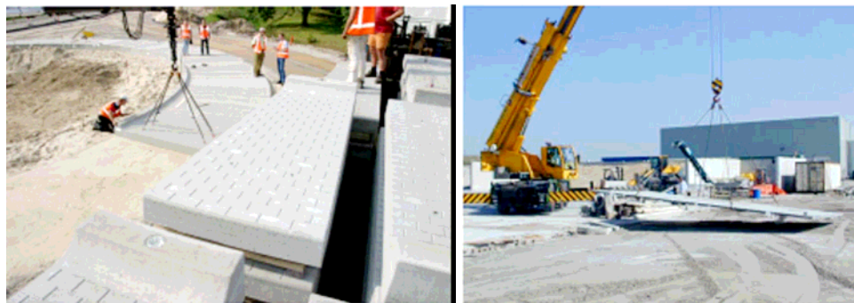
Figure 3. Precast concrete elements in a roundabout and panel lifting test in the Netherlands (12).
