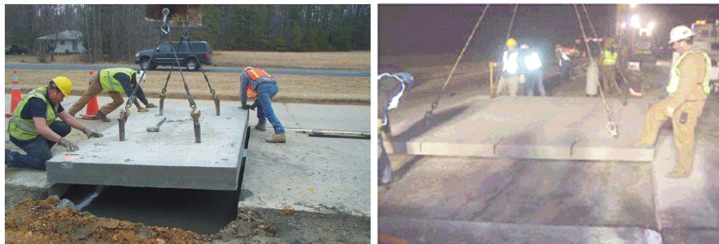
Figure 6. Precast concrete panels for experimental slab replacement in Virginia (17) and in Colorado (18).
