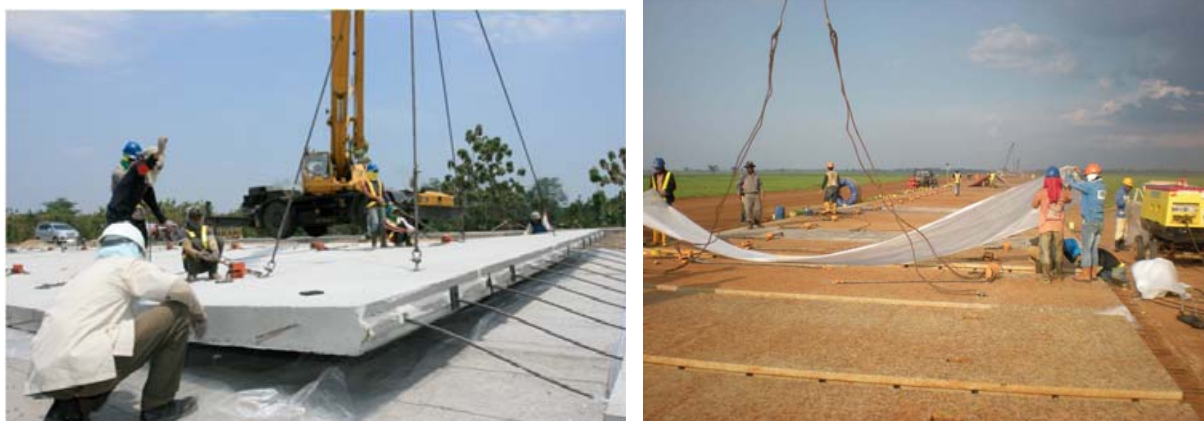
Figure 4. Indonesia PPCP installation
