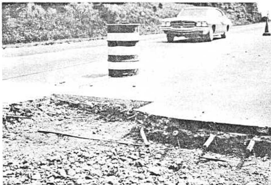
Figure 3. Incomplete full-depth restoration presents difficulty with dowel alignment.
