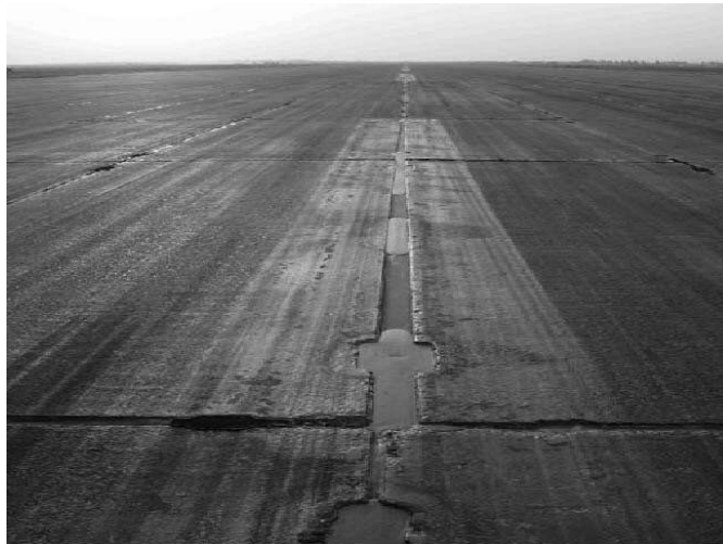
Figure 5. Opening of the centerline joint on a crowned runway thought to be due to breaking of loop welds under heavy C-17 traffic.
