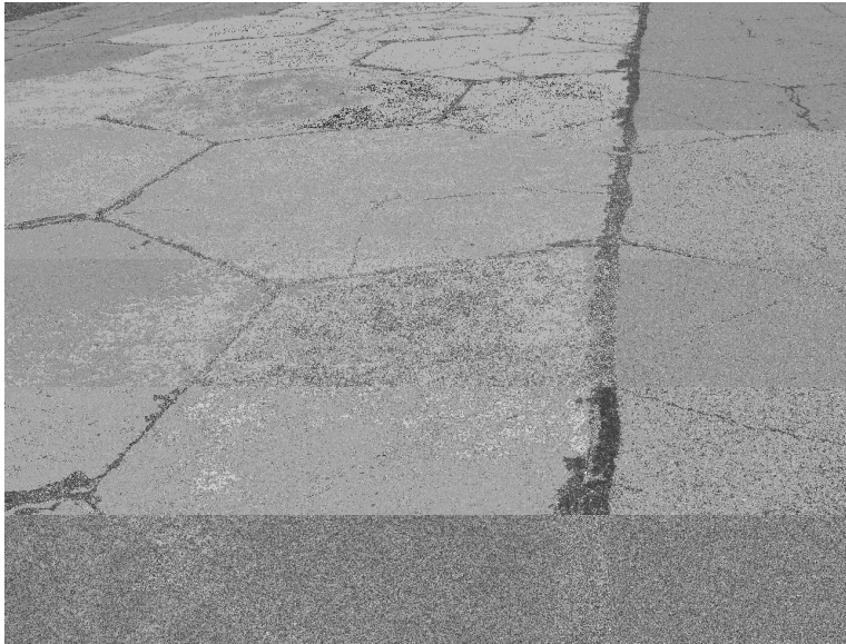
Figure 1. Example of precast unreinforced hexagonal concrete slabs on an airfield (approximately WWII era pavement and still in use).
